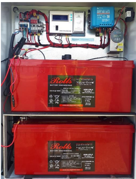
Battery Control Cabinet
